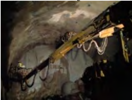
862 863 Figure B1. The drilling machine in use at a tunnel construction site
